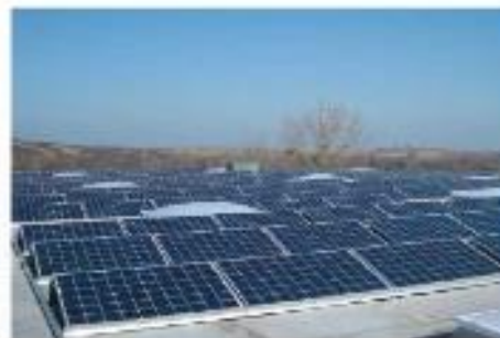
45 kWp Stadthalle Thale (Harz)
